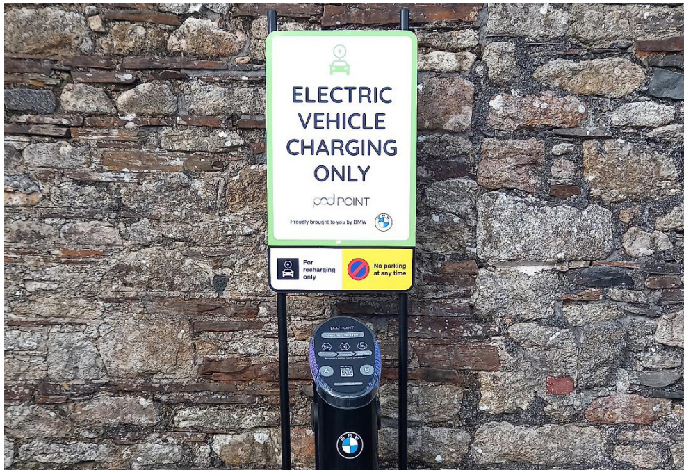
Lydford EV charger - installed in 2025
