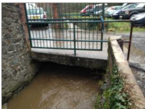
Figure 31 – First of two bridges adjacent to Auction House at south of Chuley Road site.
