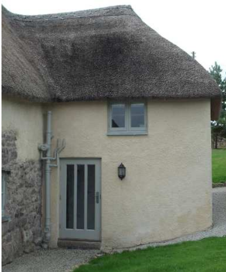
Figure 19. Discordant drainage pipes detracting from the simplicity of the rear elevation
