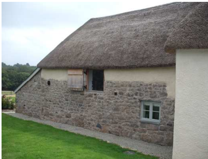
Figure 6. Middle Venton attached shippon, rear, north elevation, with approved lean-to shed/garden room extension beyond (2009 approval)
